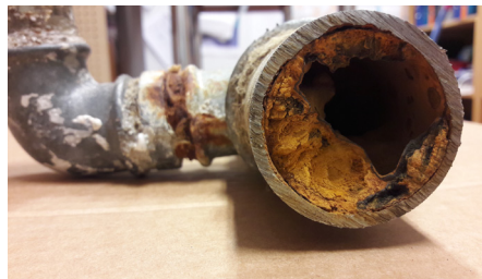
Water pipelines that are more than 50 years old can close up almost entirely, weakening water quality.
